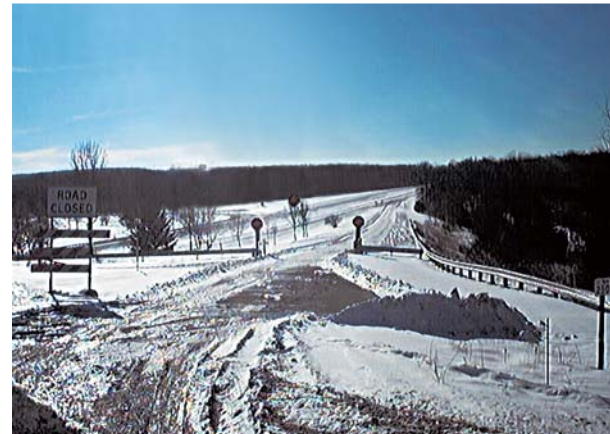
The End Of Rt. 219 As It Now Exists – Soon To Be Part Of A $50 Million Construction Project.
